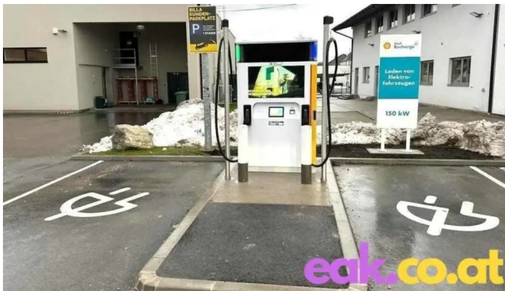
Shell recharge charging station lambach
